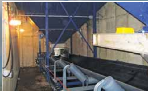
Hopper, conditioner and belt conveyor in below-grade concrete pit.
