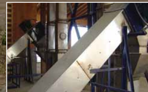
Totally-enclosed conveyor transfers conditioned material to leg.
