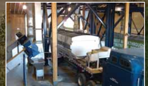
Multiple discharge lanes. Electric, telescoping dust spouts.
