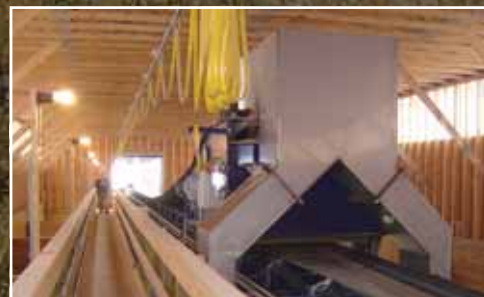
Belt conveyor with tripper discharges to bin of choice.
